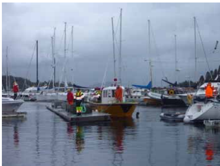
. . . to make room for another section of new pontoon tugged into place . . .
